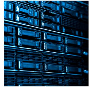
Data Center Server
